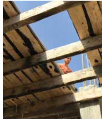
REBUILDING HOME — The wooden frame which supports the roof of Lolo's new home is slotted into place.
