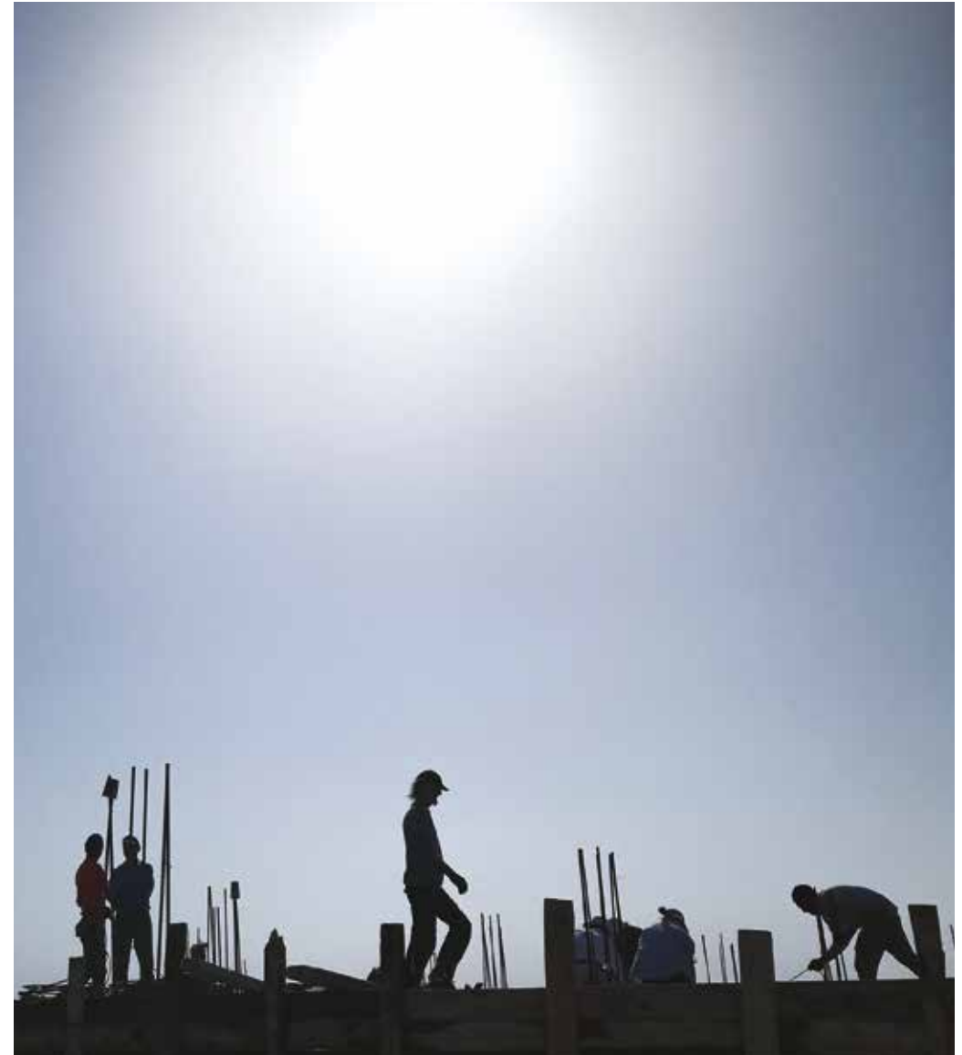
UP ON THE ROOF — Work continues on the roof of Lolo's family home. Between 2017 and 2021, just 33 building permits were given to Palestinian landowners in Israeli-controlled areas of the West Bank.
